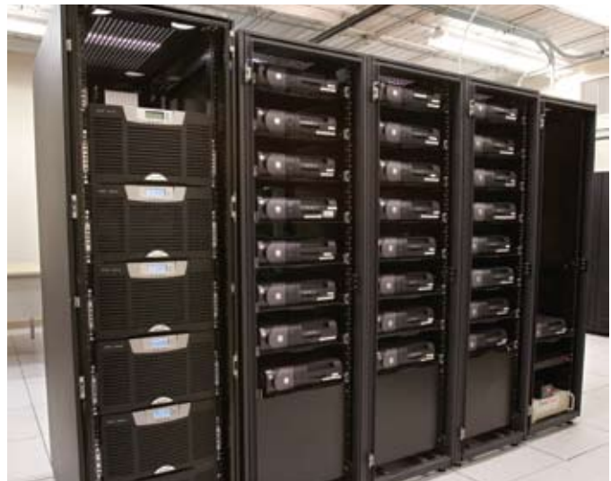
The Eaton BladeUPS remains cool even in a data centre full of servers.
