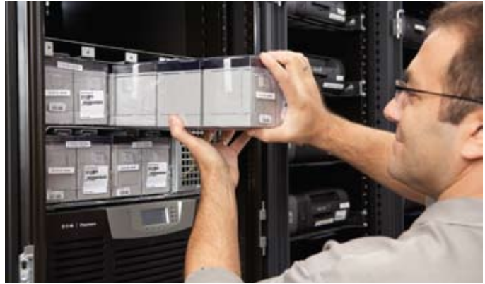
IT staff can easily replace battery modules
